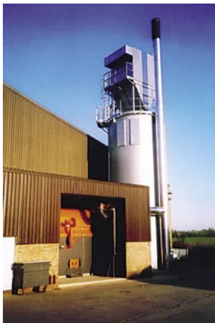
A wood burning boiler plant with a compact footprint showing the stack, silo and combustion unit.
