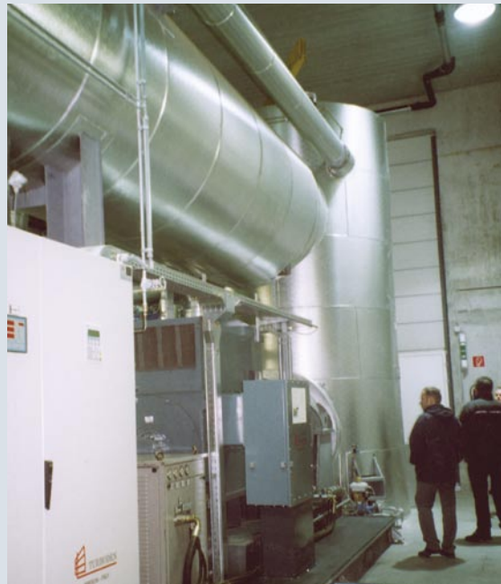
The electricity generating section of the Biostrom plant
